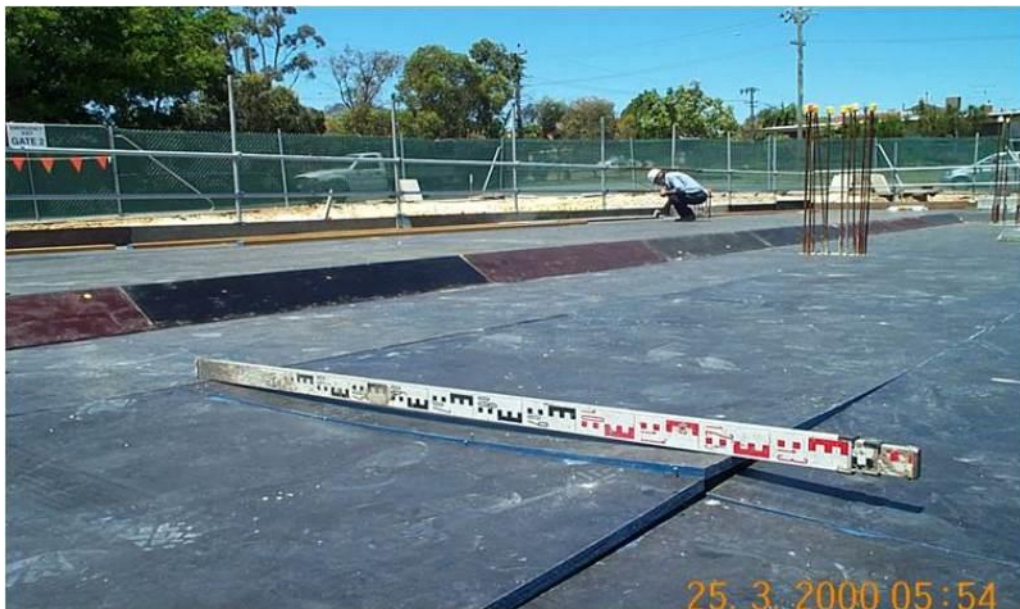
PLATE ONE: Bowed Plywood following heavy rain and hot weather
