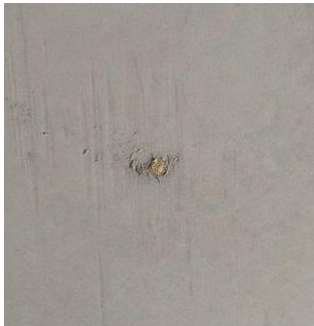
PLATE 5: Grain Imprint associated with moisture penetration at vibrator Burn
